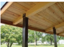
Steel Columns Powder coated steel columns
